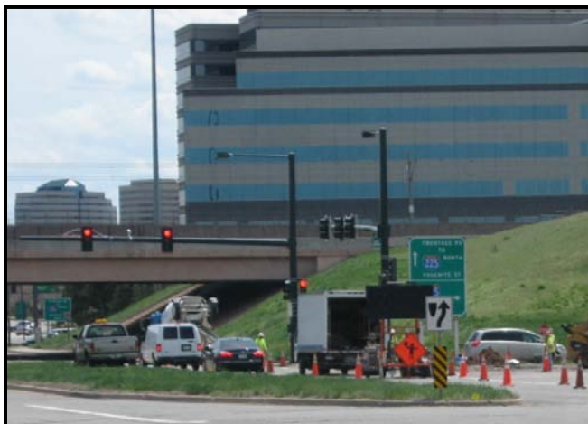
Figure 3.10 New Mast Arm Signals at DTC/Tamarac & I-225
